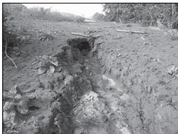
Obr. 4: Fotodokumentace výtoku č. 1 mezi patou haldy a cestou. Fig. 4: Photodocumentation of the outflow No. 1 between the base of the slag heap and the road.
