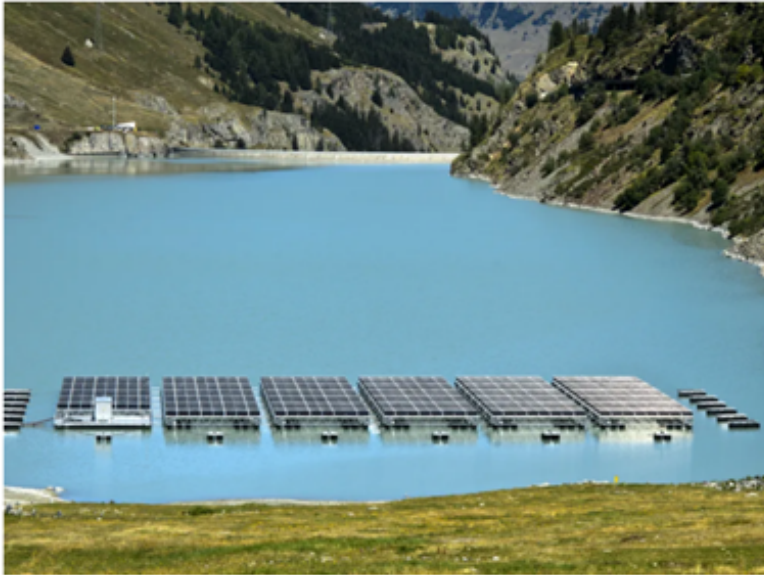
Solar panels float on a mountain lake in Switzerland. The first such system was installed in 2008. Gunter Fischer / Education Images / Universal Images Group via Getty Images
