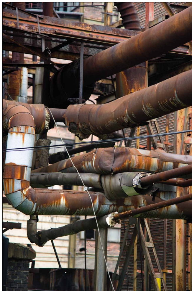
Fig. 4. Post-industrial I – National cultural monument – the blast furnaces of Lower Vítkovice. Photo: Lumír Mlčák, 2010.
